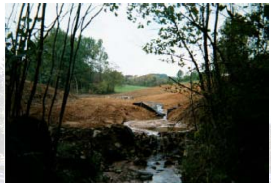
Failing ESC practices at a construction site
